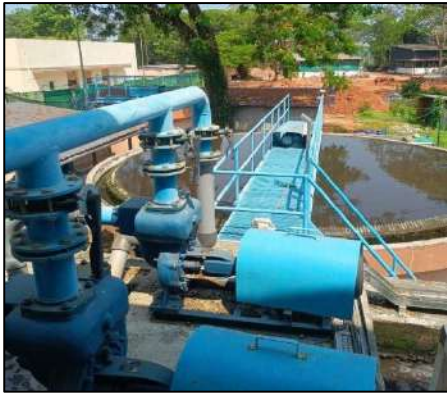
500 KLD STP at Kozhikode medical College
